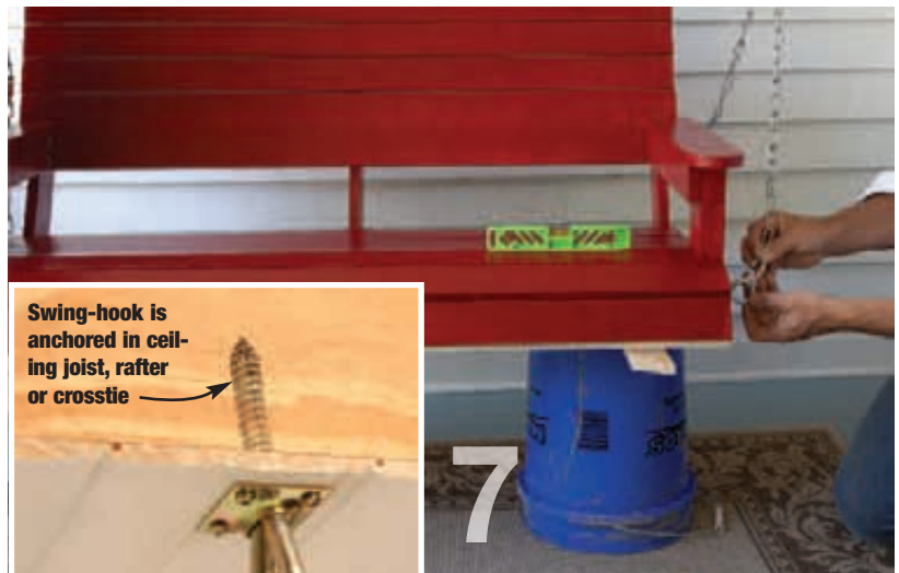
Temporarily prop up the swing at a comfortable height and angle. Use chain to connect the eyebolts to hooks that are securely anchored to framing in the ceiling (inset).
